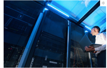
PA10 Equinix Paris Data Halls: 5,775m 2 IT Power: 12MW
