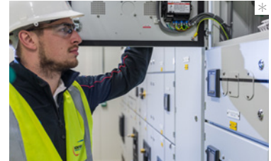
BRU01 KEVLINX Brussels Data Halls: 11,350m 2 IT Power: 32MW
